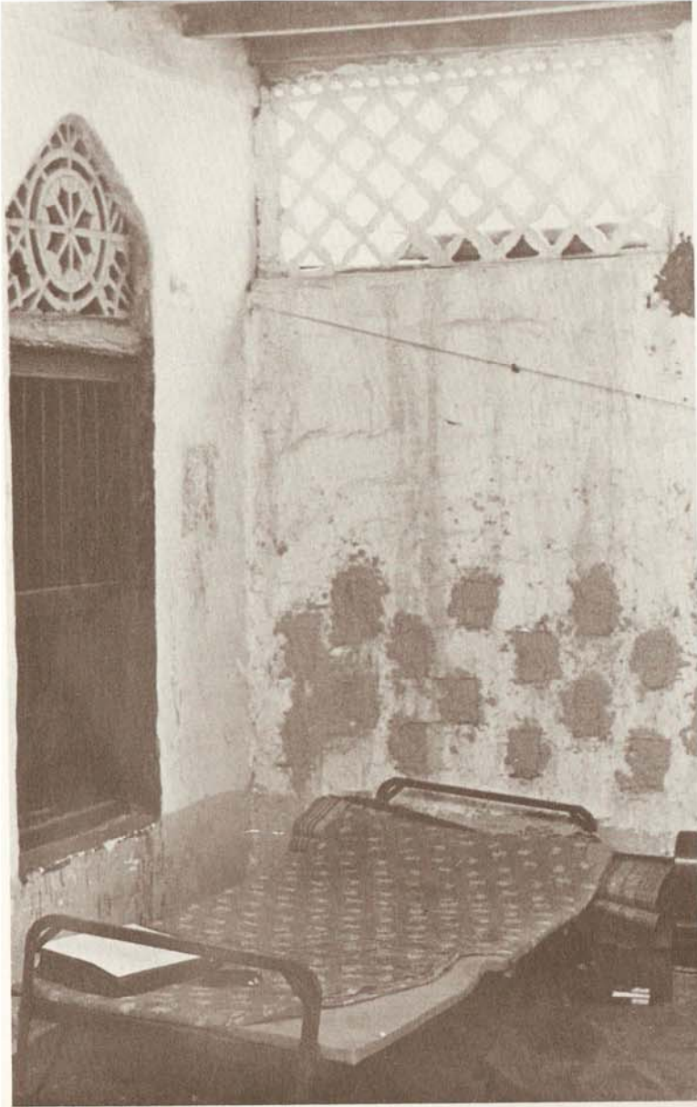
Fig. 40. Claustra in Dubai, United Arab Emirates. The claustrum at sleeping level resulted in excessive draft and had to be closed. (See p. 55.)
